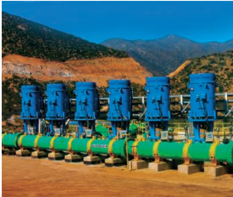
Figure 1. Reclaim water pumping system – 13,800 total installed horsepower in a copper mine in Chile
